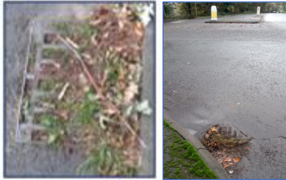
Photos show the packed drains on Holly Lane and on the upper roundabout
